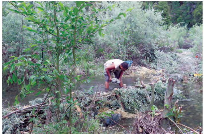
MKWC Fisheries and partners installed beaver dam analogues into Sandy Bar Creek in the summer of 2021. This photo taken on June 9, 2021, shows the human made beaver dam being built.
