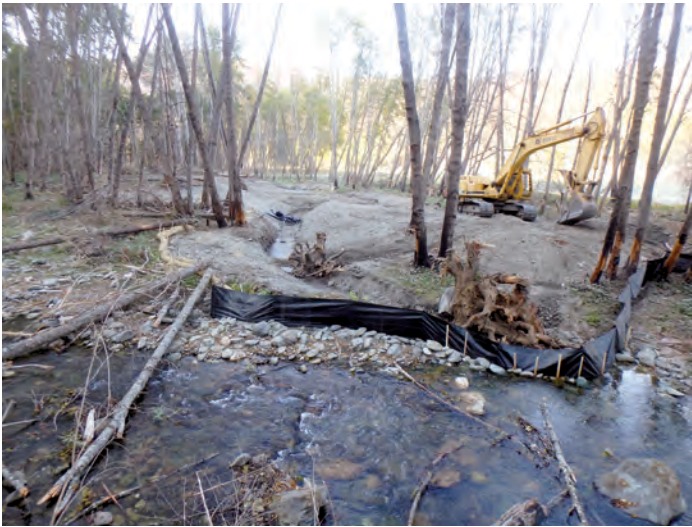
An off-channel pond being constructed on October 4, 2017. This ≈ 7,500 square foot pond was connected to Horse Creek in the fall of 2017. It provides low velocity winter rearing habitat for salmonids.
