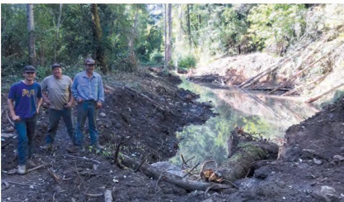
An off-channel alcove with contractor crew on September 26, 2019. This off-channel alcove is connected to China Creek.
