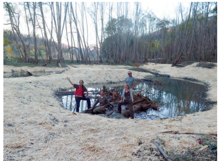
MKWC's Fisheries and Plants personnel happy to have completed mulching the banks of the newly excavated pond connected to Horse Creek. This pond has been utilized every winter since it was created by at least 500 salmonids. The salmon are seeking refuge from the adjacent creek, which has high velocities during winter and spring.
