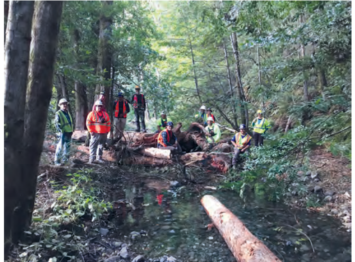
MKWC Fisheries partnered with the Karuk Tribe, the Yurok Tribe, the U.S. Forest Service, and the California Department of Fish and Wildlife to install 24 wood structures into Aikens Creek in the summer of 2020. Pictured here is the implementation crew on one of those installed wood structures on August 13, 2020.
