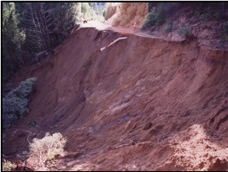
Figure 31. Road failure on Ukonom Ranger District.
