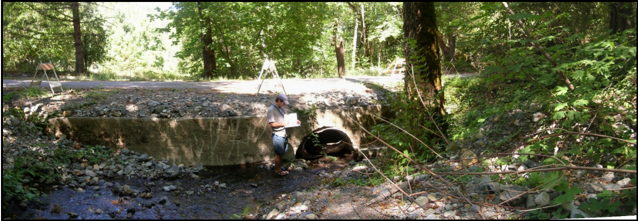
Figure 9. China Grade Road crossing on Little Horse Creek failed in 2006 Flood and was replaced with a bridge in 2008.
