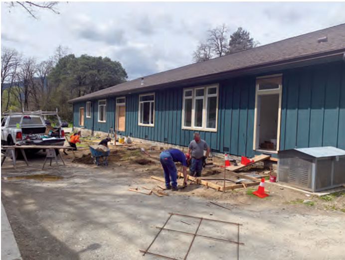
KJ Construction pouring footing for the new back deck. By Michael Stearns
