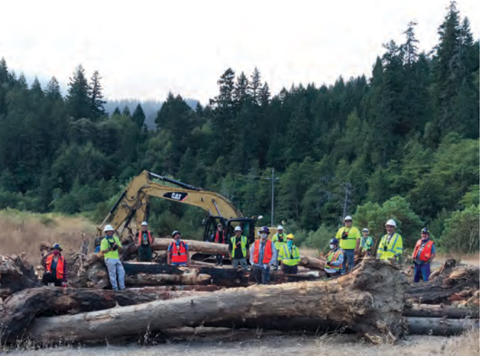
August 11, 2020. On the ground implementation crew on one of the stockpiles of logs that were added to the creek, to benefit Klamath Basin fish, wildlife, and plants. All photos this article by MKWC Fisheries, unless noted
