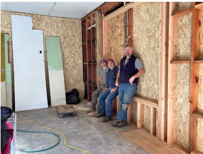
Many thanks to KJ Construction, who have been doing a great job on the remodel! By Blythe Reis
