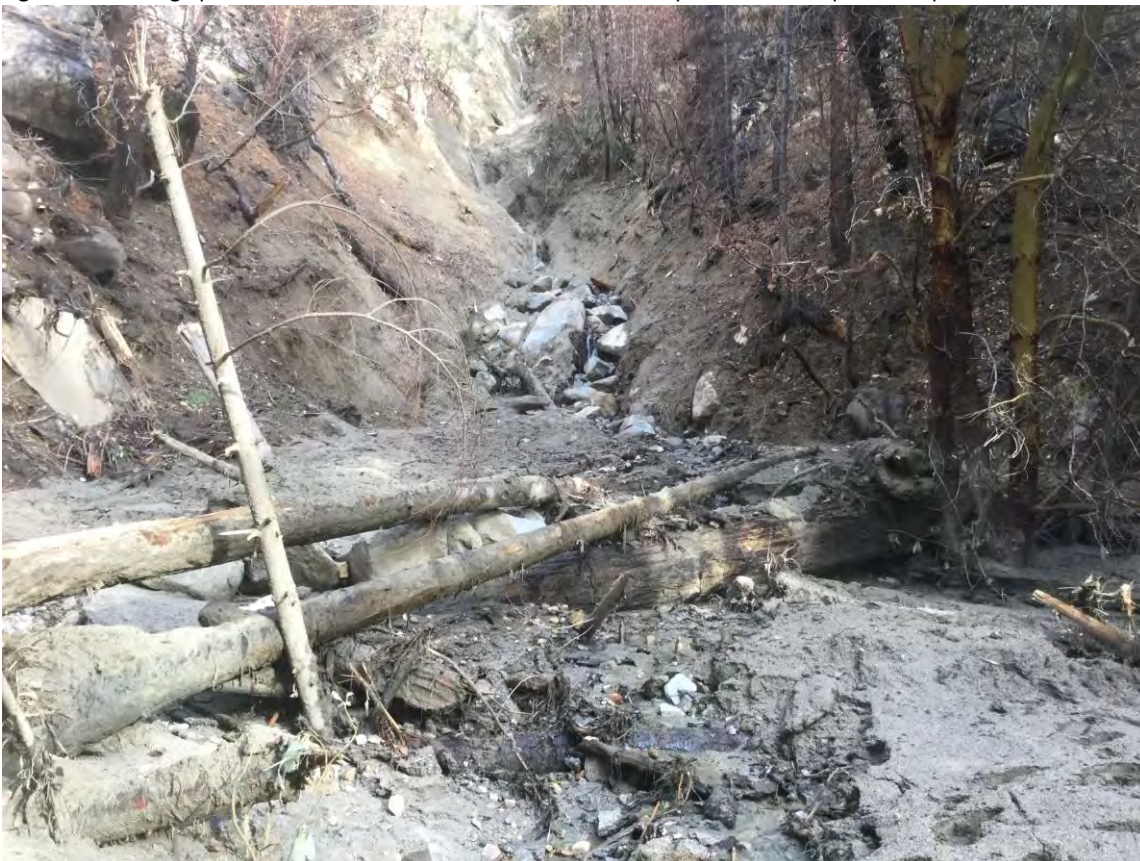
Figure 20. Looking upstream at eroded channel from 13N11. Taken by Adam Dresser prior to repair.
