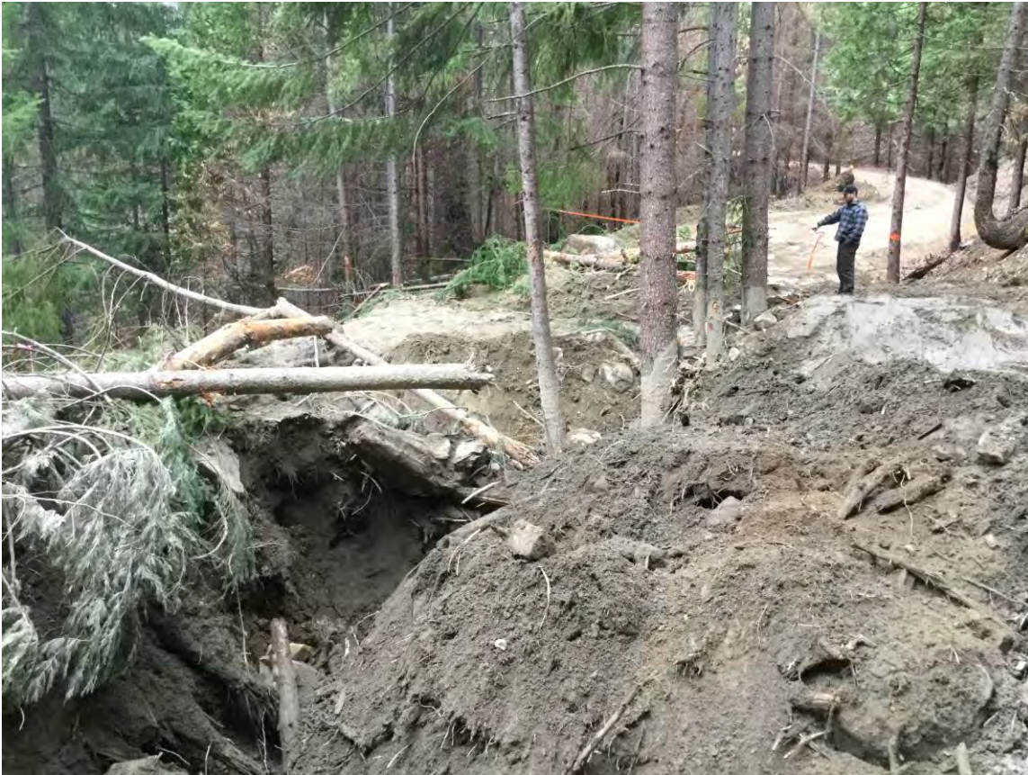
Figure 18. 13N11 buried by failed debris post repair to restore flow.
