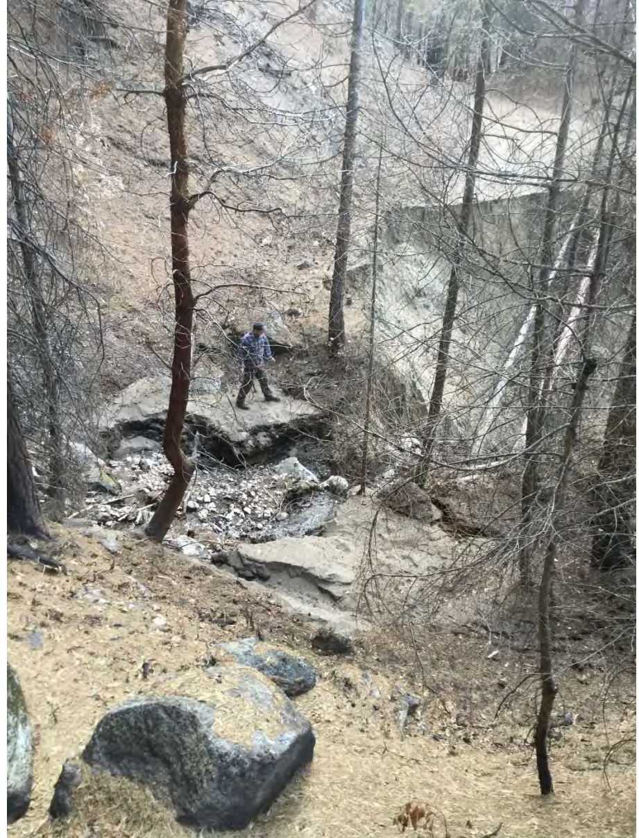
Figure 4. Overview of sediment filled inlet basin.
