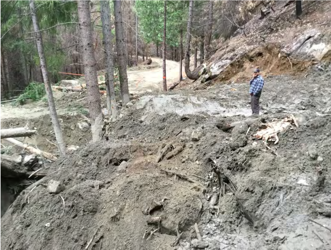
Figure 19. 13N11 buried by failed debris post repair to restore flow.
