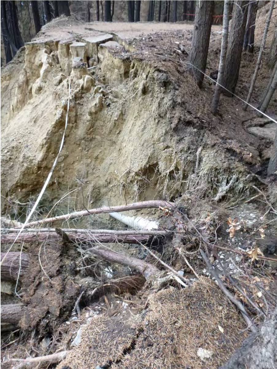
Figure 3. View of right scarp near top of 15N17 failure showing in place culvert with buried inlet. Inlet is roughly to the right (as viewing photo) of the base of downed trees about 1.5-2 feet below surface of deposited sediment.
