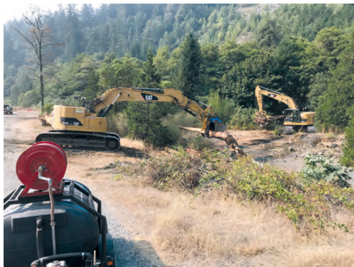
Yurok Tribe excavator operators, Seagull and Roger, bringing in wood for the most upstream structure
