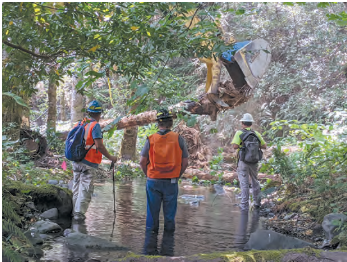
Fish biologists from the Karuk Tribe, Yurok Tribe, and Six Rivers National Forest, guide placement of logs in Aikens Creek by Yurok Tribe excavator operator Roger Boulby.
