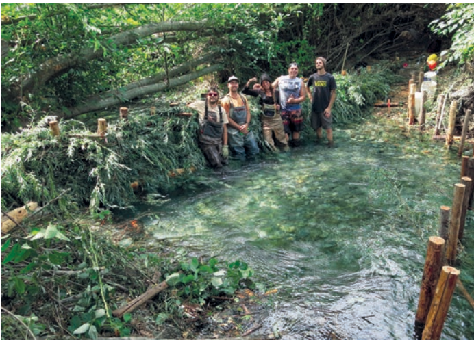
MKWC Fisheries Crew (top) weaving willow around Douglas-fir posts. Celebrating a job well done (above).
