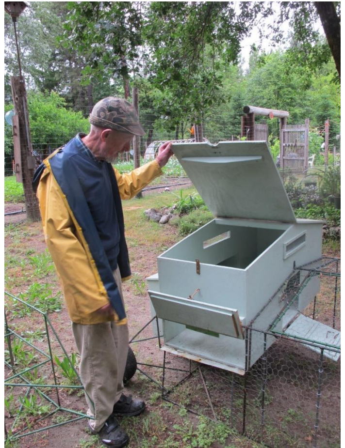
4. Add hinges and latches to doors. Note that only one side of the roof is hinged.
